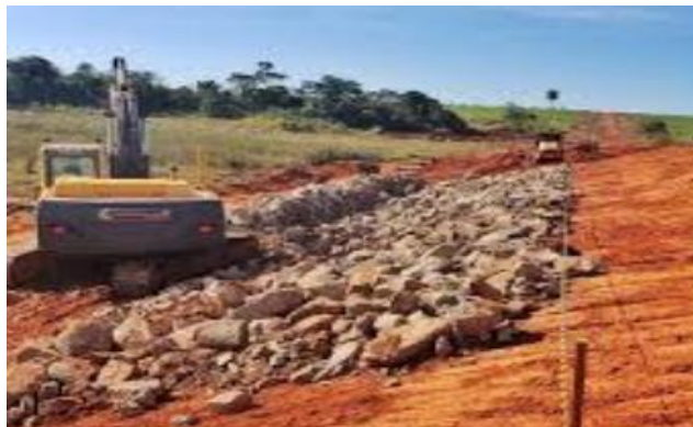
Figura 13 - Rip-Rap. Fonte: https://www.facebook.com/inframataengenharia/posts/2424748267564708
