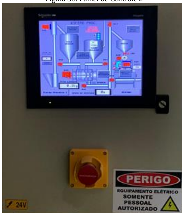
Figura 30: Painel de Controle 2
