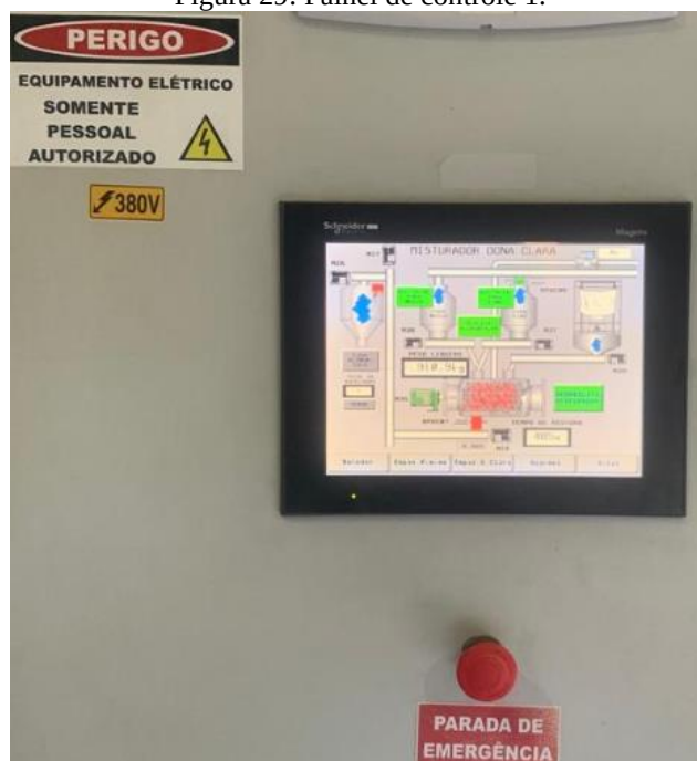
Figura 29: Painel de controle 1.
