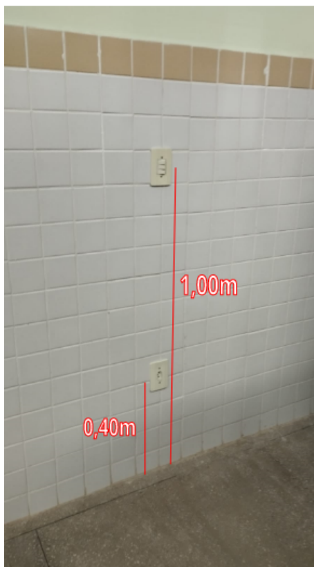
Figura 18: Interruptor e tomada
